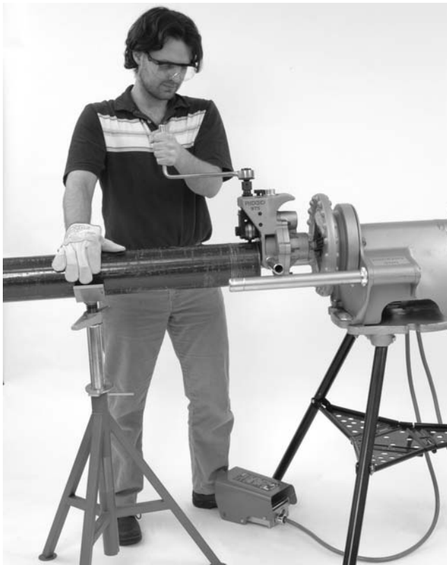
Figure 13 – Applying Force To Pipe While Grooving To Maintain Tracking
