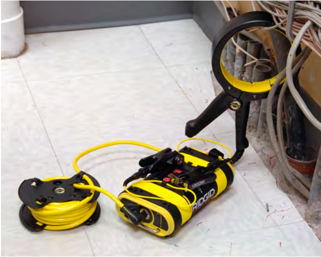
Figure 11 – Inductive Clamp in use
